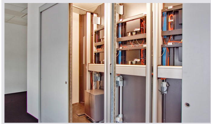
Sliding doors on the back of the large display screen cladding as room-in-room function. Behind the sliding doors are the stable display racks for holding the LC displays.
