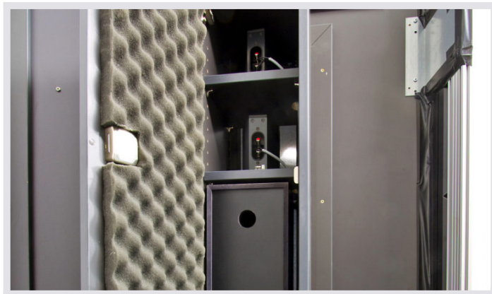
Speaker installation behind the large display screen cladding. Media cabinets with two adjustable shelves and two LSG all-glass doors.
