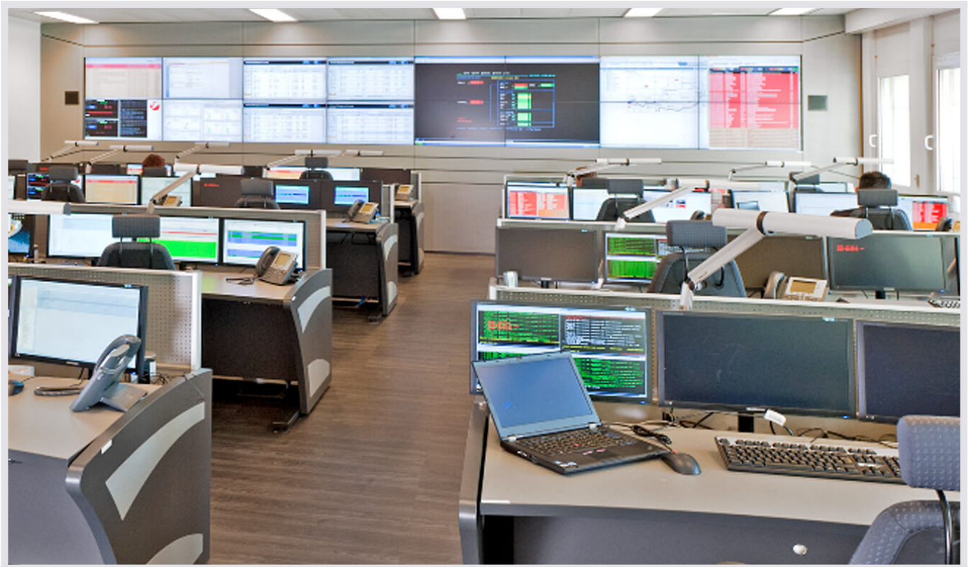
UniCredit Vienna. Control room from JST
