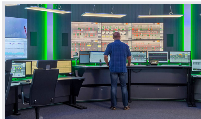
Workstation in control room with height-adjustable desk.
