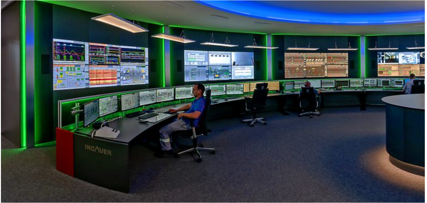
Virtual 360° tour through the control room.
