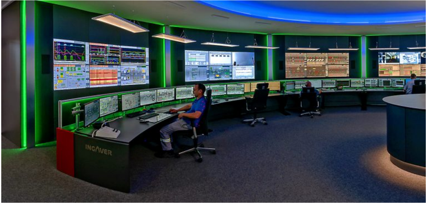
Virtual 360° tour through the control room.
