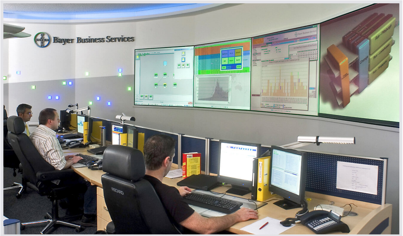
Control center of the Global Data Center in Leverkusen
